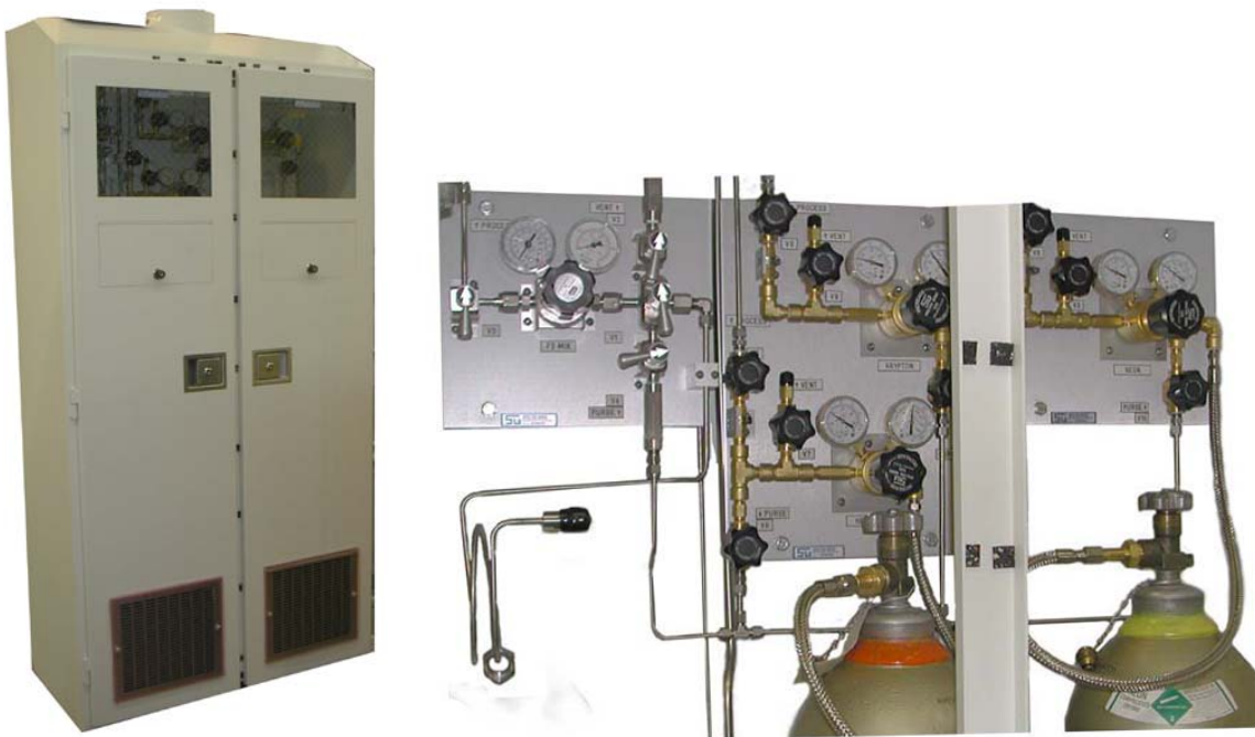
Figure 5-7. Gas Cabinet and Gas Panel
